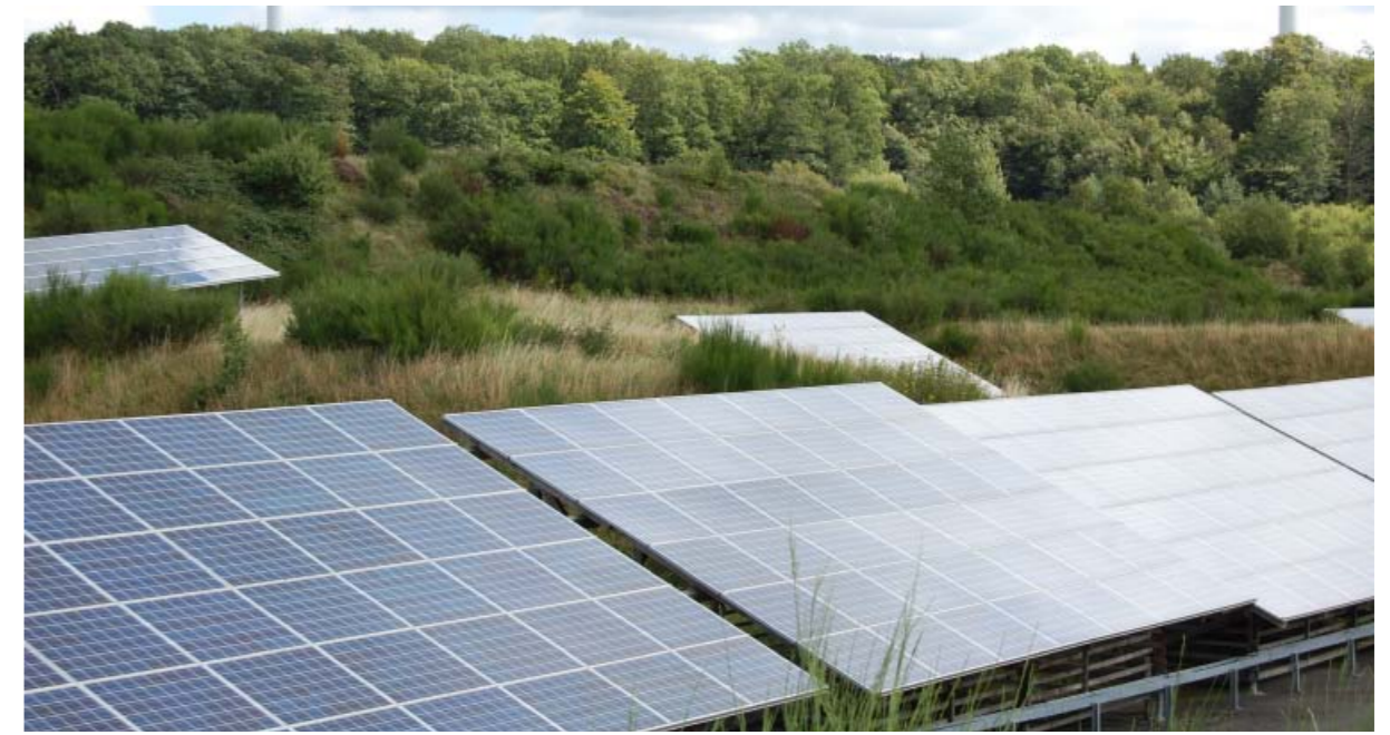
Photovoltaic modules in solar parks can be integrated into a wide range of landscapes without dominating them. (Photo: Renewable Energies Agency)
