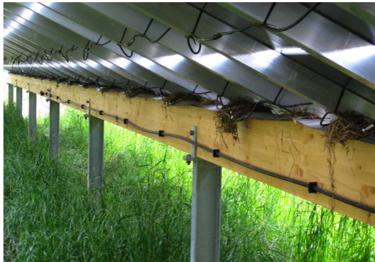
The module supports serve as nesting places for birds. (Photo: BELECTRIC)
