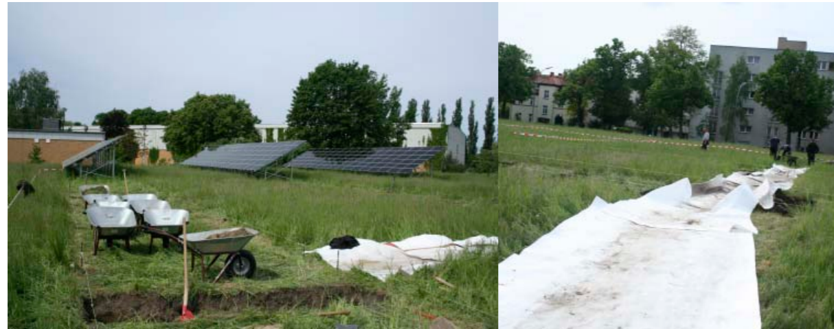
Wheelbarrows were used to remove excavated earth during the building work on the Tegel waterworks site. Because of the high ecological value of the sites, protected plants were transplanted and geo fleece was used to minimize trampling damage (right). [Photo: Tim Peschel]
