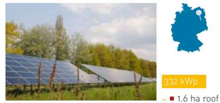
Berlin-Tegel waterworks solar plant Solargruppe Nord (S.G.N.), completed 2009
